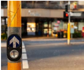
Pedestrian operated signals
